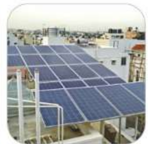
SOLAR ROOF TOP SYSTEM
